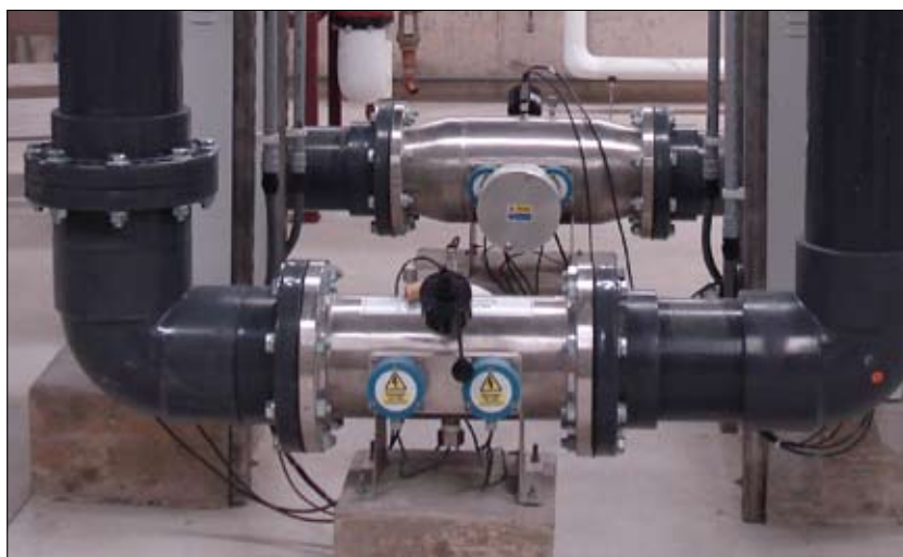
ETS chambers installed vertically in pool filter room
